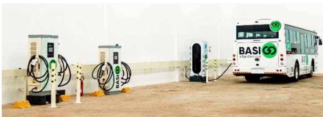
Credit: BasiGo e-Bus Charging Station
